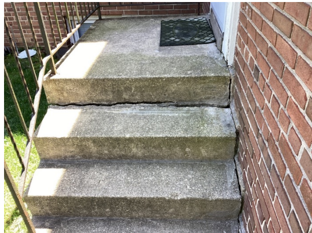
Stair settlement and cracks
