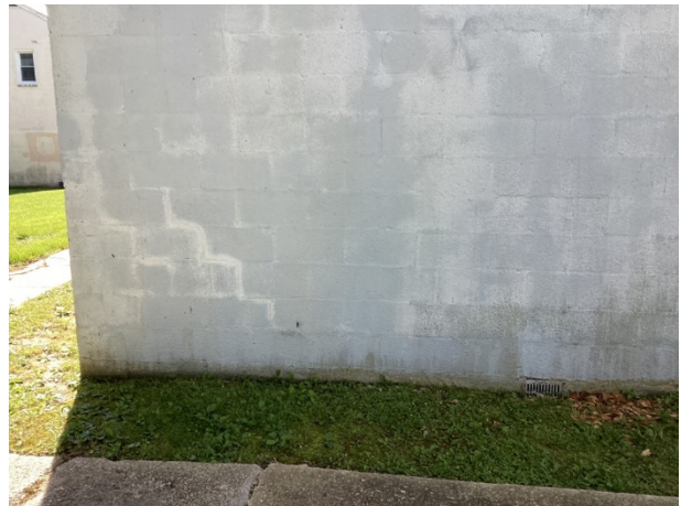
CMU cracks and staining
