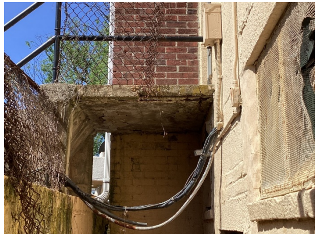
Exposed rebar at underside
