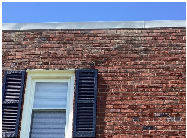
Rust jacking and steps cracks
