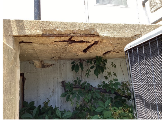
Exposed rebar at 3851 26 th Avenue
