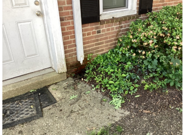
Loose fastener and improper drainage
