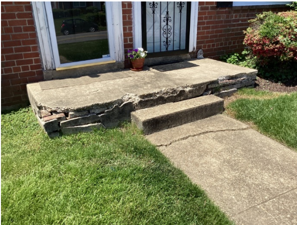
Concrete stoop overview with spalls
