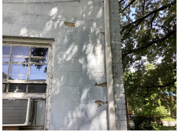
CMU spalling spalls
