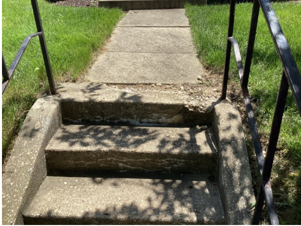
Concrete stairs deterioration
