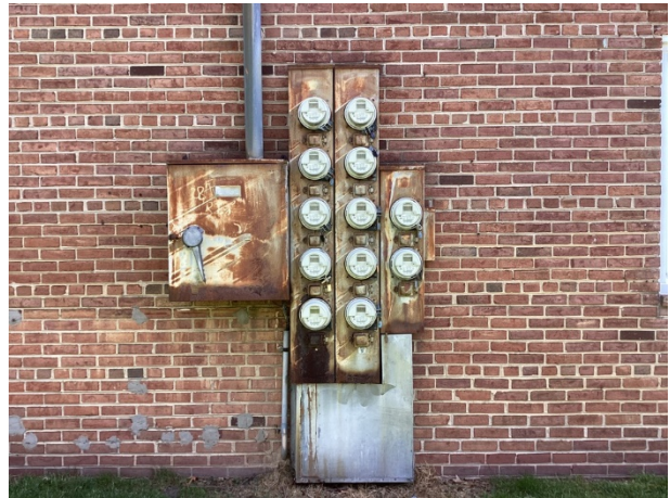
Meter stack overview with rust
