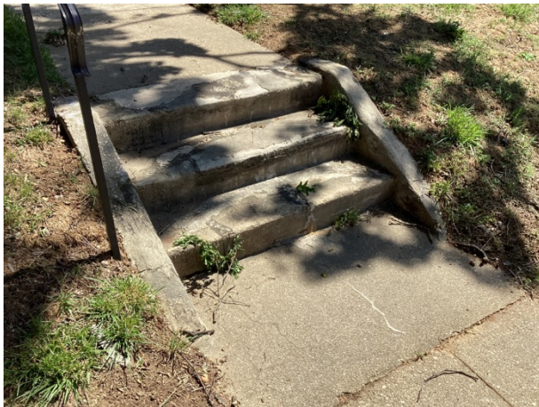
Concrete stair overview with scaling
