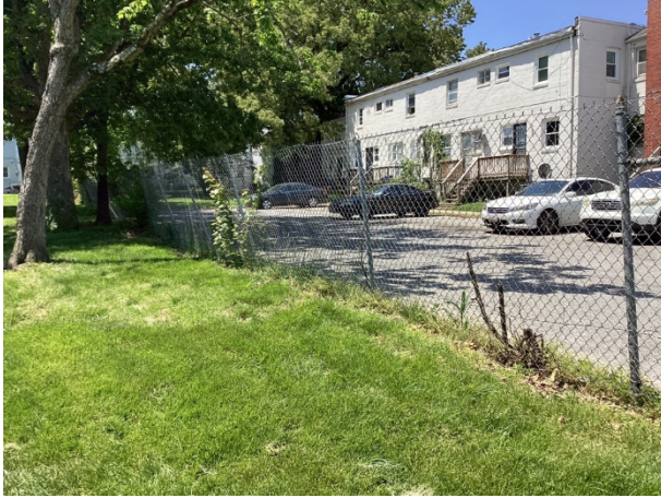
Chain link fence with leaning sections
