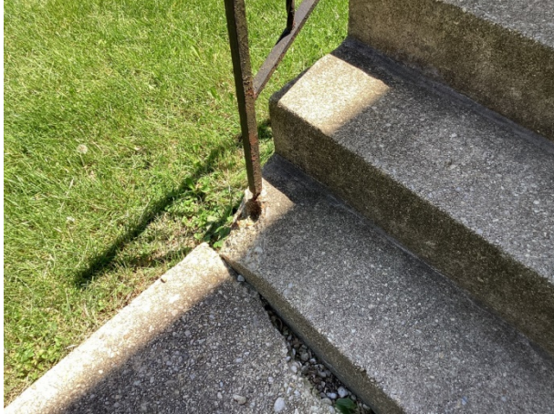
Metal railing rust
