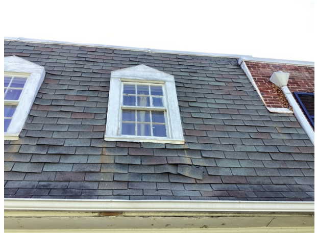
Loose and curled shingles
