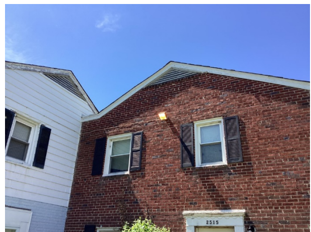
Security light fixture
