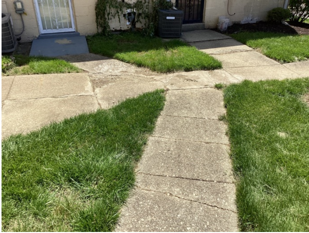
Concrete sidewalk overview with scaling
