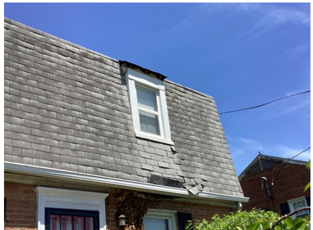
Shingle failure and exposed insulation
