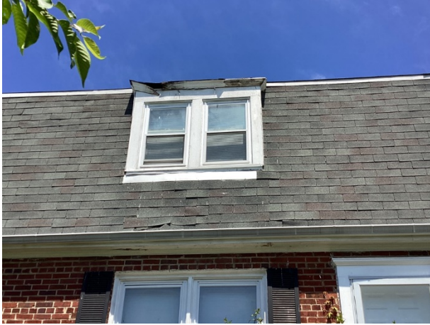
Shingle curl and fascia damage
