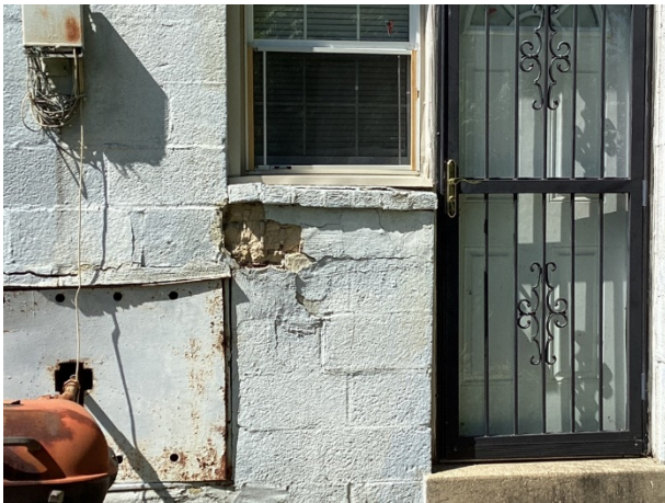
CMU cracks and spall
