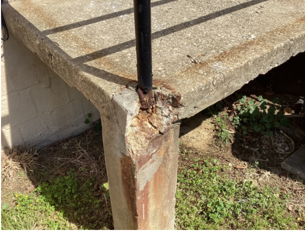
Concrete spall with rust
