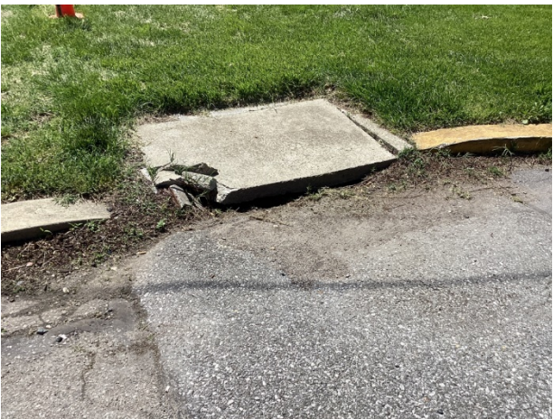
Catch basin settlement
