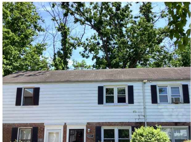
CMU cracks and staining
