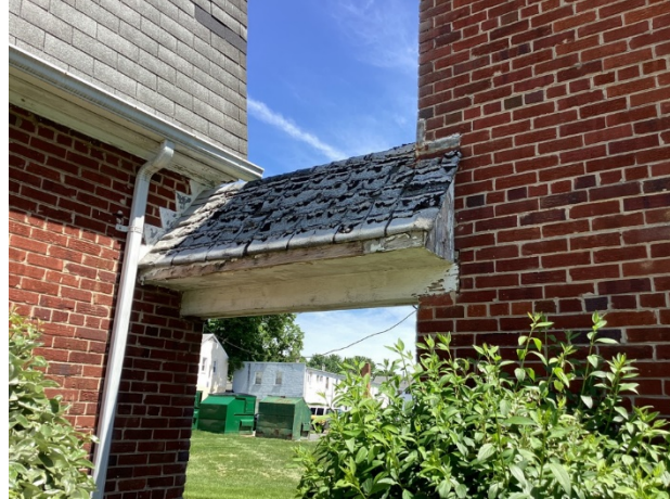
Breezeway roof deterioration
