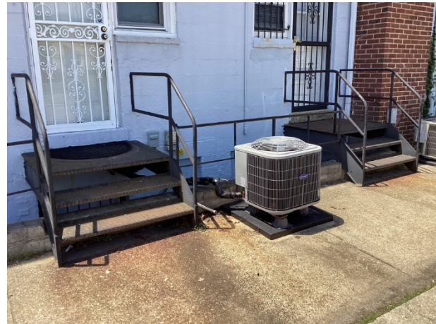
Metal steps near 3918 25 th Avenue
