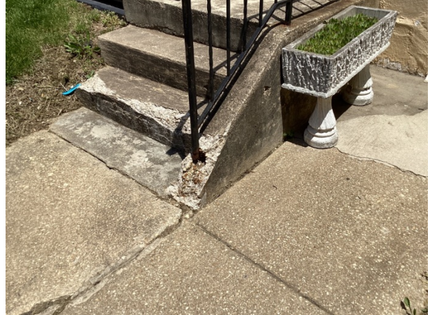
Metal railing rust
