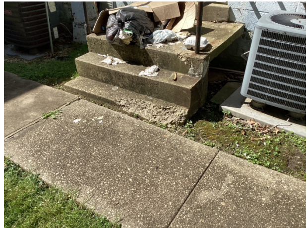
Concrete stoop cracks
