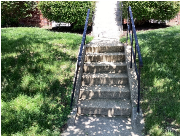
Steel railing overview with leaning section at 2504 Iverson Street
