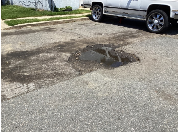
Pavement pothole formation
