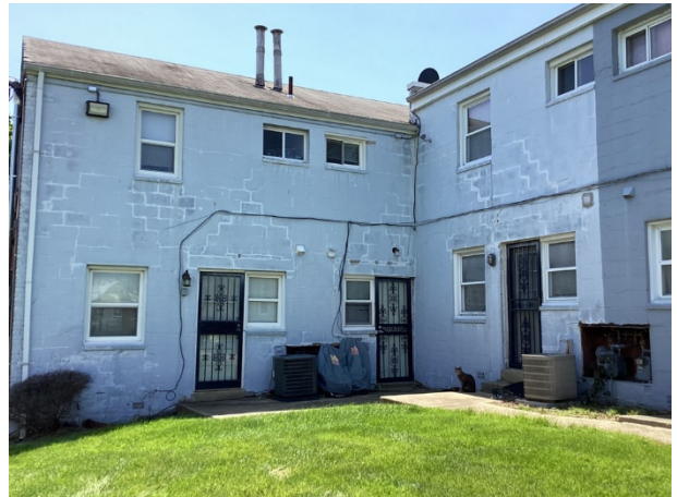
CMU cracks and finish deterioration
