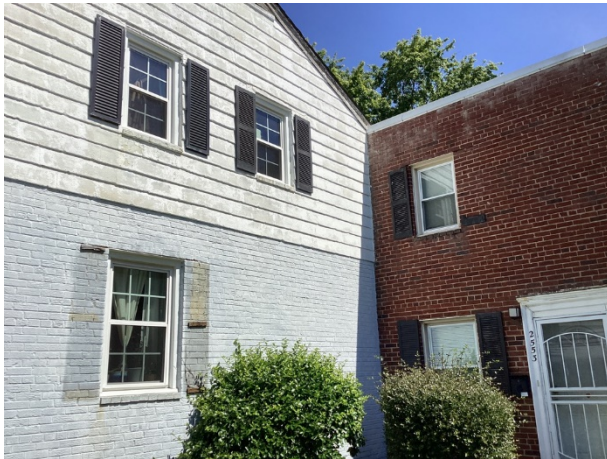
Vinyl shutters with missing and damaged shutters
