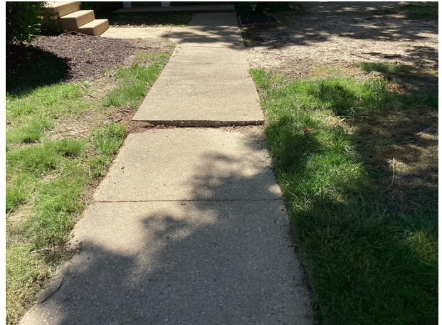
Sidewalk trip hazard near 3902 25 th Avenue
