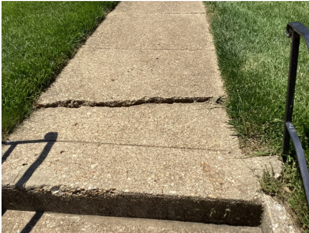
Sidewalk trip hazard near 3859 26 th Avenue
