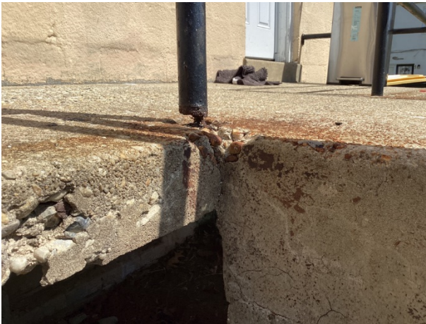
Railing rusted through
