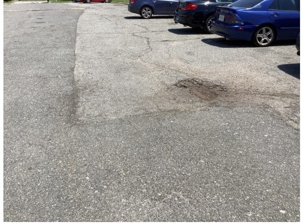
Asphalt pavement parking lot overview with cracks
