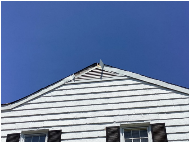
Missing fascia board
