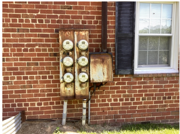
Meter stack overview with rust
