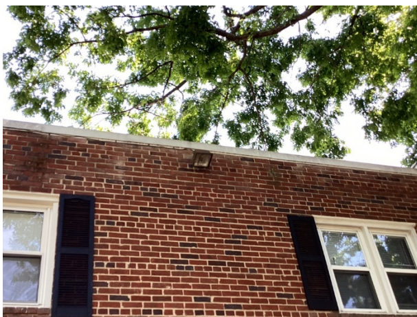
Security light fixture
