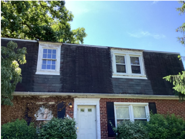
Staining and organic growth
