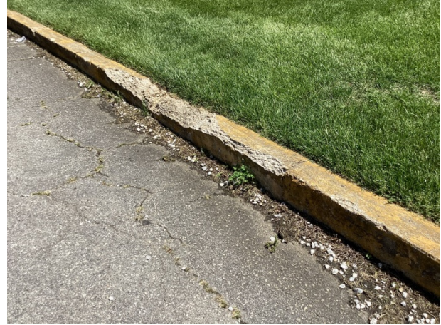
Concrete curb spall
