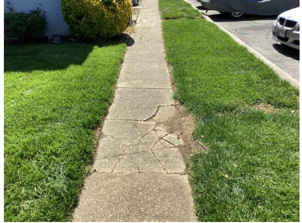
Concrete sidewalk overview with cracks
