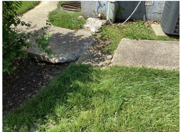
Sidewalk cracks and undermining
