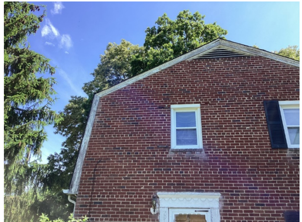
Wood fascia deterioration
