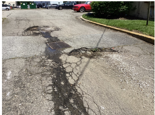
Pavement pothole formation
